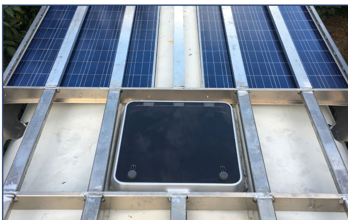
Solar panels in their retracted position.
