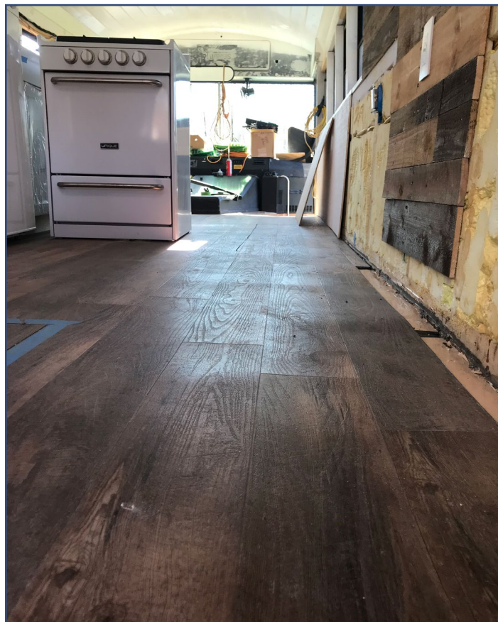
Warped flooring with some added relief cuts.
